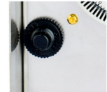
Magnetic circuit breaker on secondary to protect lighting system
